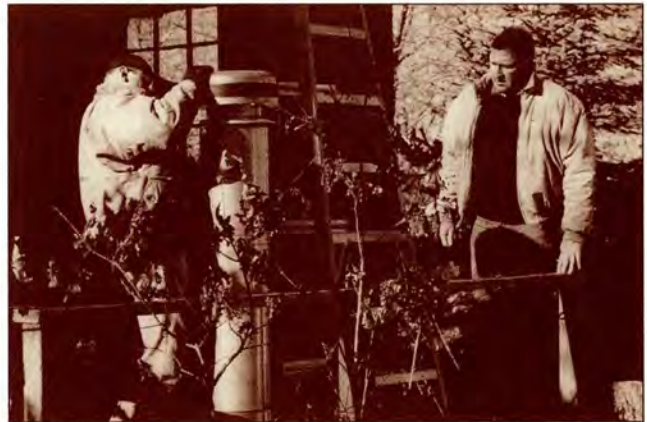
Special thanks to Mrs. Pat Beck who donated a wood stove for the Trust's management cabin at Berglund Preserve. Shown installing the stove are (l. to r.) Parker Hough of Hough & Guidice Realty, and Maurice Skerritt of Skerritt Construction.
